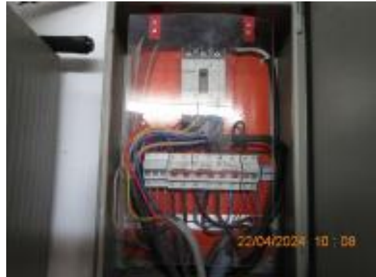
26. Inner cover for electrical panel.JPG
