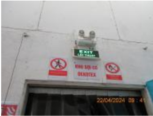
15. Emergency light and exit sign.JPG
