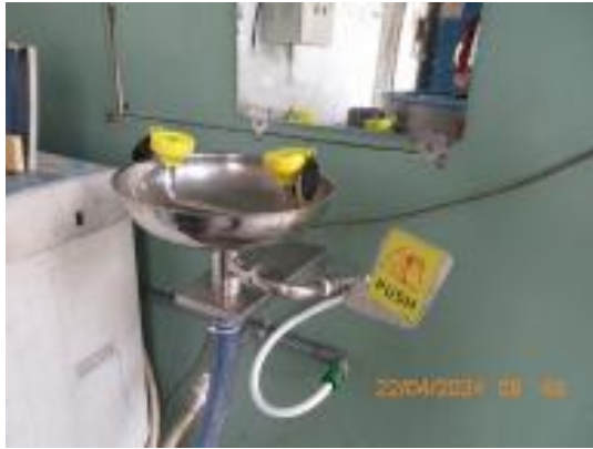
33. Eye wash station.JPG
