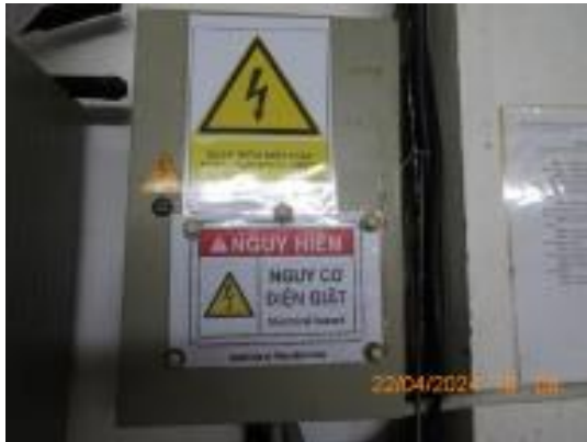
25. Warning sign and safety cover for electrical panel.JPG
