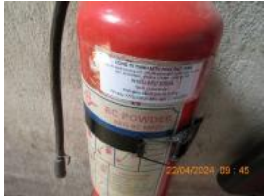
24. External inspection record for fire extinguisher.JPG
