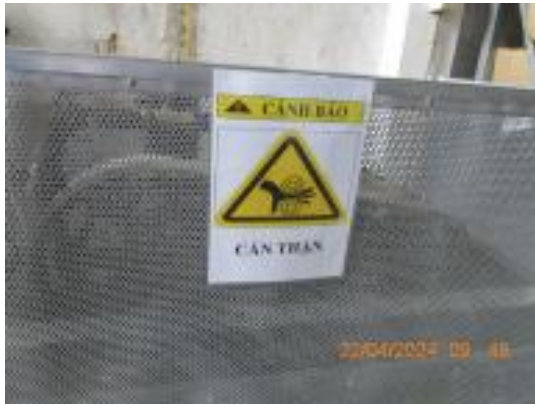
31. Safety warning sign.JPG
